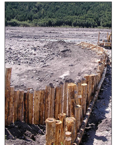
4. Install pile dikes to form pilot channels throughout the lower basin to create sinuosity for the sediment to be captured by the dikes.
